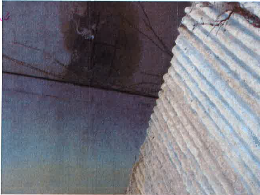
DECK PANEL BAY "B" ABUT. #1 SPALL & EXP. STL
